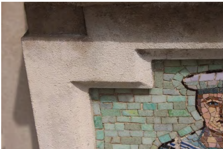
3.3 Eroded pointing and missing mosaic tesserae
