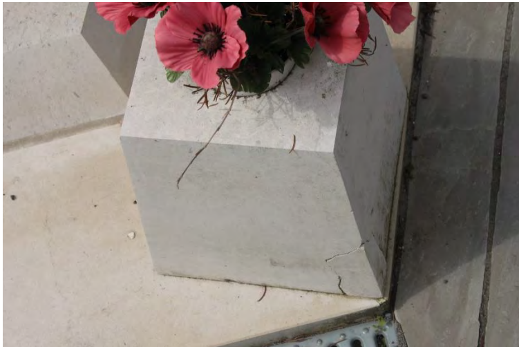
2.1 Damage to edge of stone flower vase
