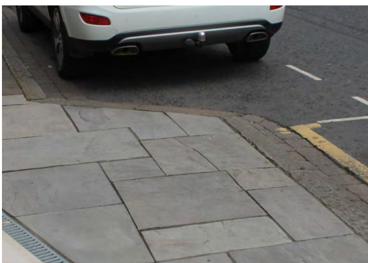
I.3 Fractured paving flags by kerb
