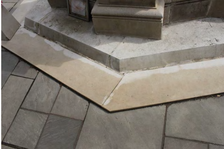
I.1 Uneven joints, and salt staining to paving stones
