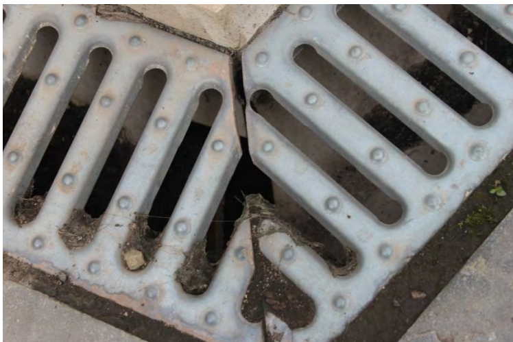
I.2 Unsupported edges and flimsy material to ACO grating.
