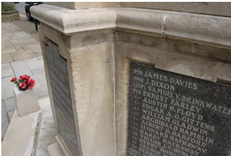
2.2 Eroded stone mouldings and face
