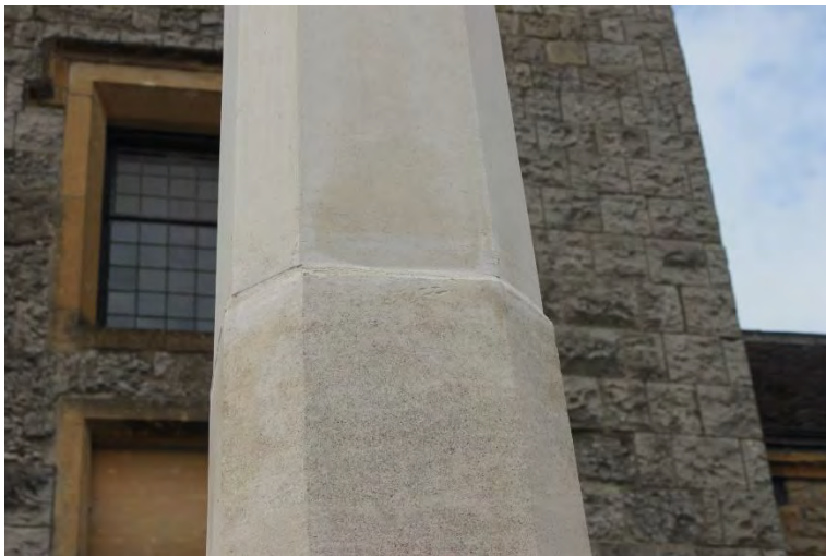
3.2 Inadequately shaped new stone
