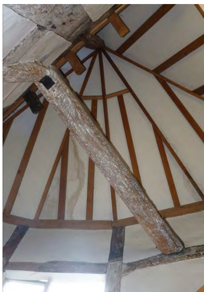
Fig 10.5 Worsening dampness in ceiling and timber frame wall at junction of Painted Room stairwell with north west corner of main building.
