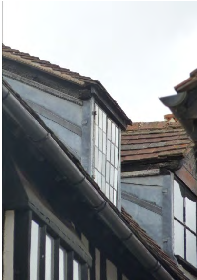
Fig 1.1 Fractured verge pointing at junction of south east roof with main building. Mastic pointing to lead flashing pulling away.
