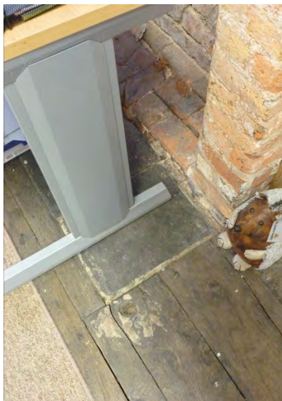
Fig 13.3 Dampness in south external wall to first floor office.
