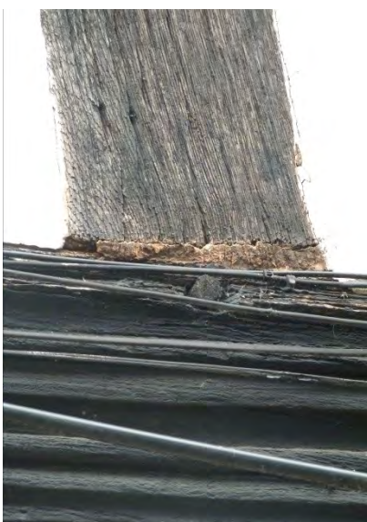
Fig 5.3 Gaps to timber frame beneath window cill, south elevation.
