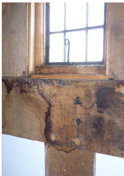
Fig 12.5 Water penetration to north pitch beneath Velux rooflight.
