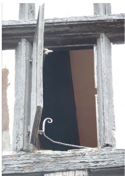
Fig 7.3 North dormer window frame in poor condition. Gaps allowing water entry around dormer carpentry.
