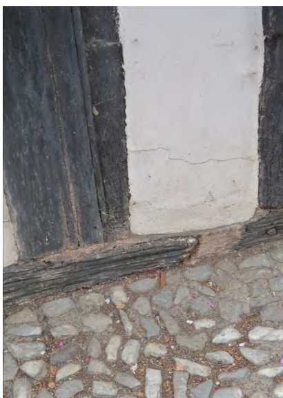
Fig 6.5 Cellar hatch, loose cobbles and sets, allowing water penetration.
