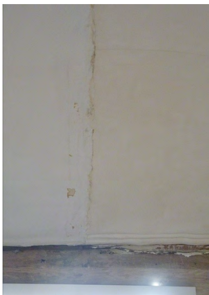
Fig 9.1 Historic plaster suffering fractures and mechanical damage in eastern ground floor office.
