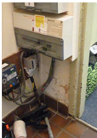
Fig 8.3 Active leaks to chimney flue in easternmost ground floor office.
