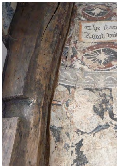
Fig 15.5 Hairline cracks in repairs to Painted Room plasterwork.
