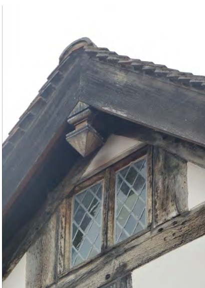
Fig 6.3 West gable carpentry would benefit from staining. Pigeon roosting on pentice board.
