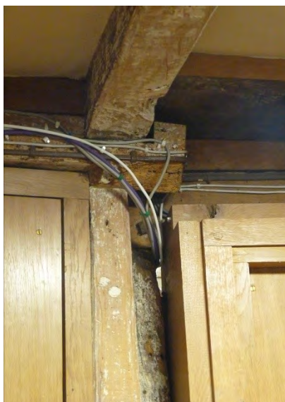
Fig 10.1 Dampness in ceiling between kitchen and rear passage G5.
