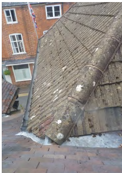
Fig 12.1 Dampness adjacent to east attic dormer.
