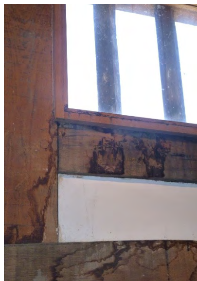
Fig 13.5 Ill-fitting windows and carpentry in poor condition, to south facing windows.
