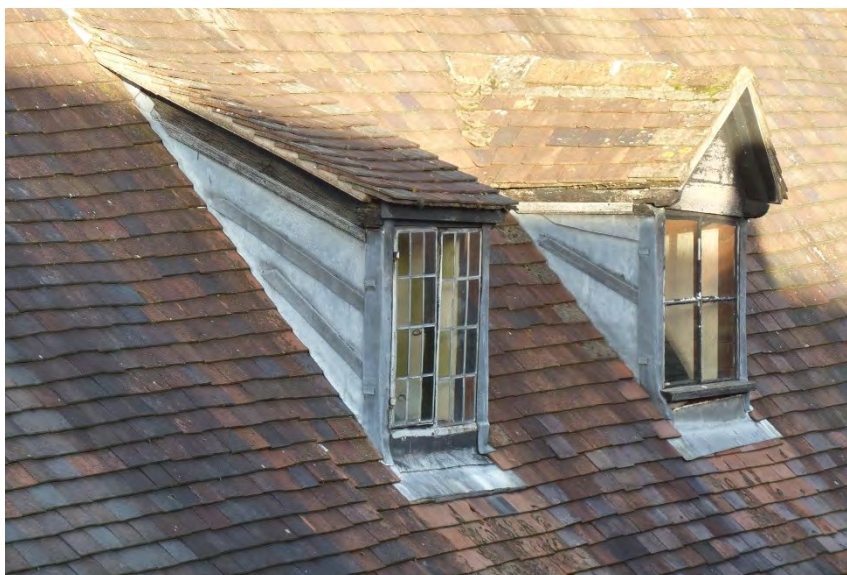
Fig 3.3 and 3.4 Slipped clay plain tiles with moss build-up, windows and roof carpentry to south dormers in need of overhaul. Slipped apron flashings beneath dormer windows.
