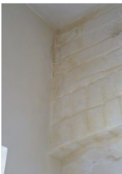
Fig 9.5 Water staining to modern timber frame to Painted Room stairwell.
