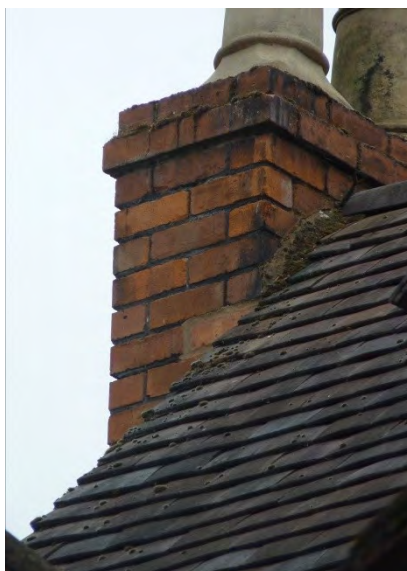
Fig 4.2 North elevation of central stack. At least one friable brick. Moss grows on joints between slate capping and on brickwork.
