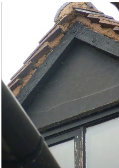
Fig 2.1 Sapling growing at north east junction with British Legion. Moss building up at roof abutments with British Legion wall.
