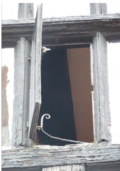
Fig 8.1 First floor window in poor condition with putty failing.
