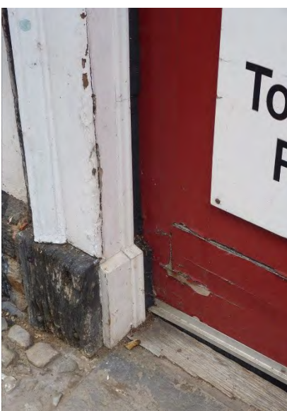
Fig 7.5 Painted hardwood bay window in need of maintenance.
