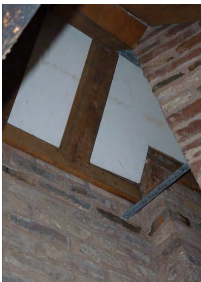
Fig 12.3 Small areas of dampness in attic adjacent to central stack.
