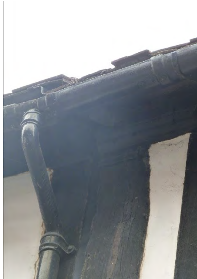
Fig 1.3 Decaying bituminous felt and window frames to east dormer, south elevation.
