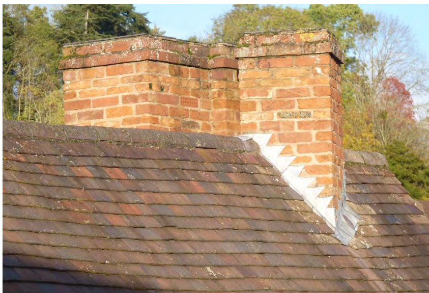
Fig 4.1 Central chimney stack. Upper brick courses and slate and cement capping saturated. Mortar bedding to ridge tiles loosening.
