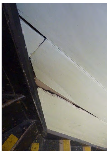
Fig 15.1 Timber ground floor set on damp, loose stone walls to cellar.
