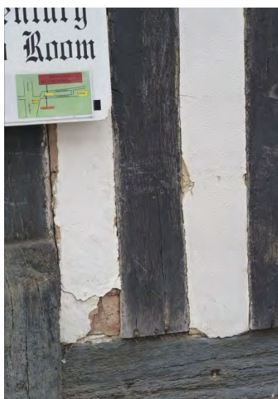
Fig 5.5 Fracturing to first floor infill panel to timber frame.
