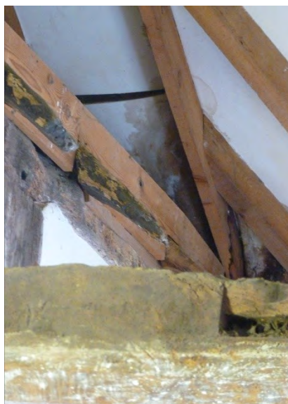
Fig 11.1 Worsening dampness in north timber framed wall.
