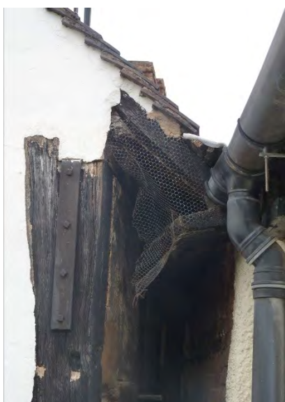
Fig 2.5 East end roof overwhelmed with tree branches and leave mould. Fractured verge pointing and open end to eaves carpentry.
