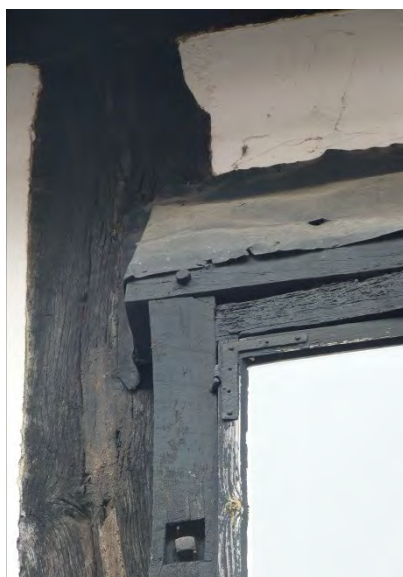
Fig 5.1 Rainwater staining to rafter ends beneath eaves. North west corner.
