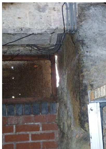
Fig 15.3 Damp cellar walls at south west corner beneath timber frames and floor beams.
