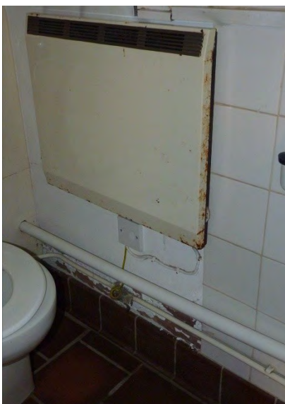
Fig 10.3 Dampness in south wall above sole plate, to reception.
