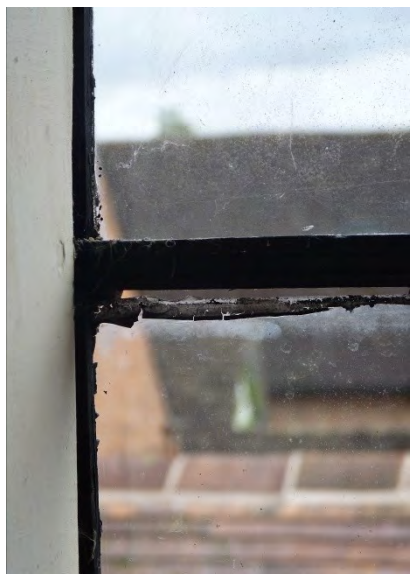
Fig 11.5 Dampness in ceiling adjacent to south wall of Pink Room.
