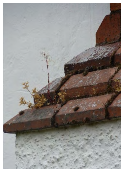
Fig 2.3 Gaps where rainwater enters at junction of head of lean-to roof with timber frame and render, south east corner.
